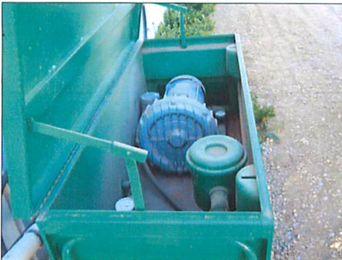
PHOTO 2 View of Soil Vapour Extraction System.
