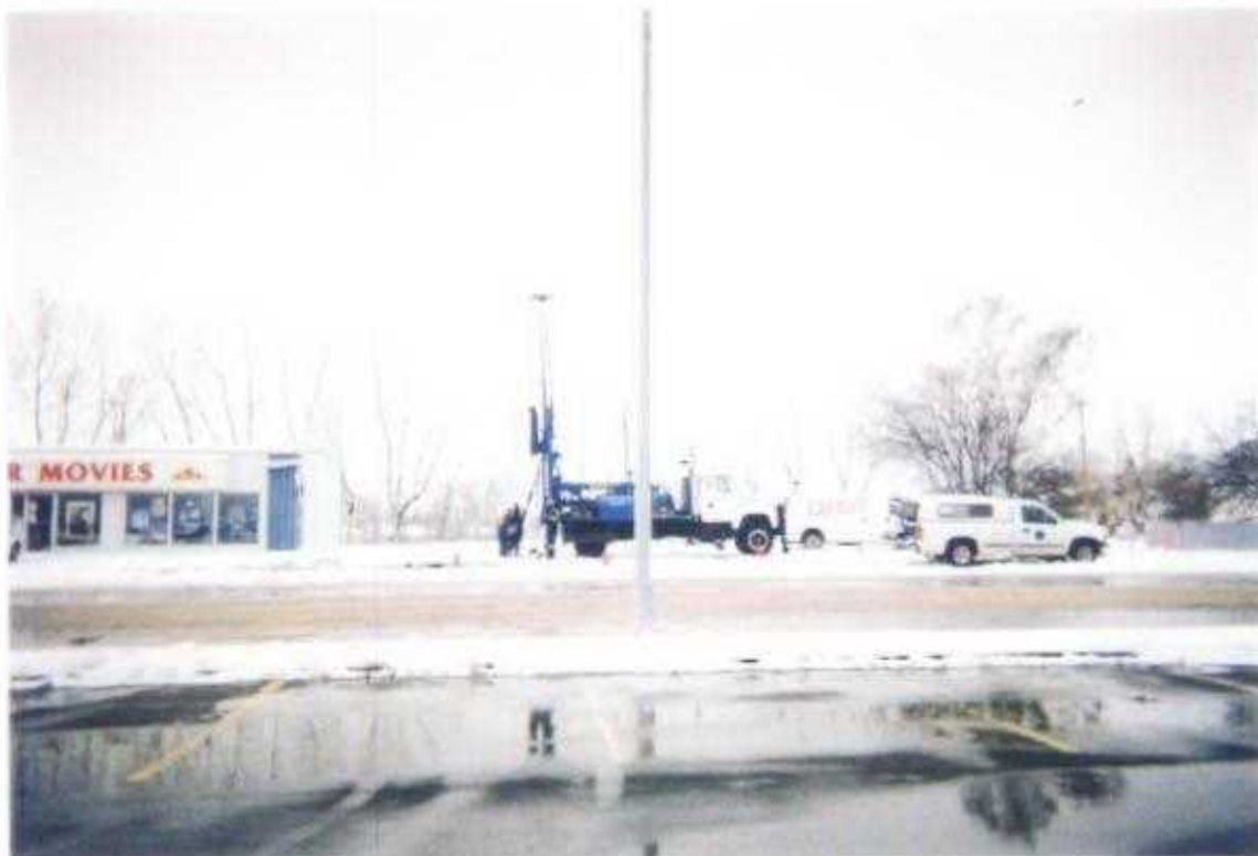
Photo No. 10: May 6, 2002; Phase II Hydrocarbon Environmental Site Assessment Lots 5 & 6, Block 28, Plan 3845 CO; 419 - 10 th Avenue, Carstairs, Alberta Looking West. Drilling Borehole #3.
