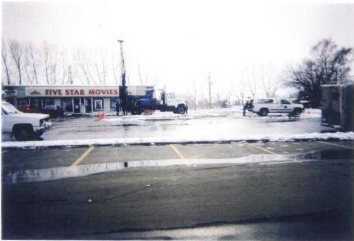
Photo No. 14: May 6, 2002; Phase II Hydrocarbon Environmental Site Assessment Lots 5 & 6, Block 28, Plan 3845 CO; 419 - 10 th Avenue, Carstairs, Alberta Looking West. Drilling Borehole #8.
