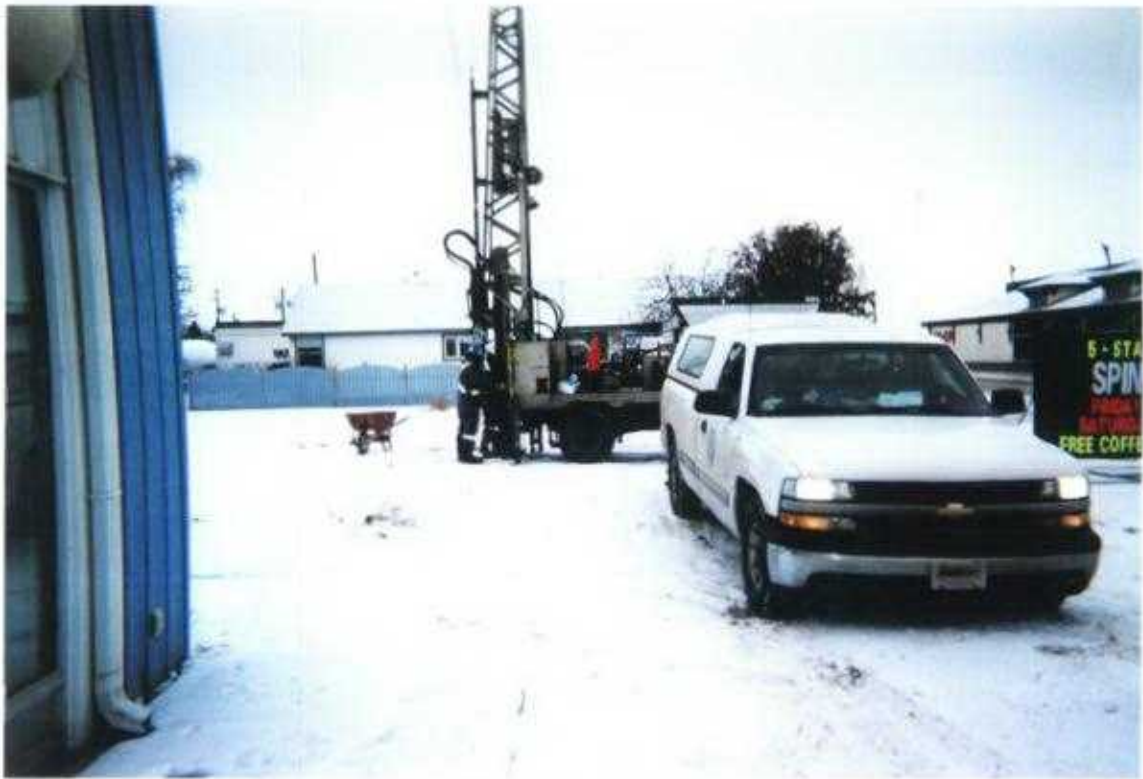
Photo No. 1 January 15 & 16, 2003; Phase III: Hydrocarbon ESA-Delineation Lots 5 &6, Block 28, Plan 3845 CO; 419 - 10 Avenue, Carstairs, Alberta Looking North. Drilling Borehole #9.
