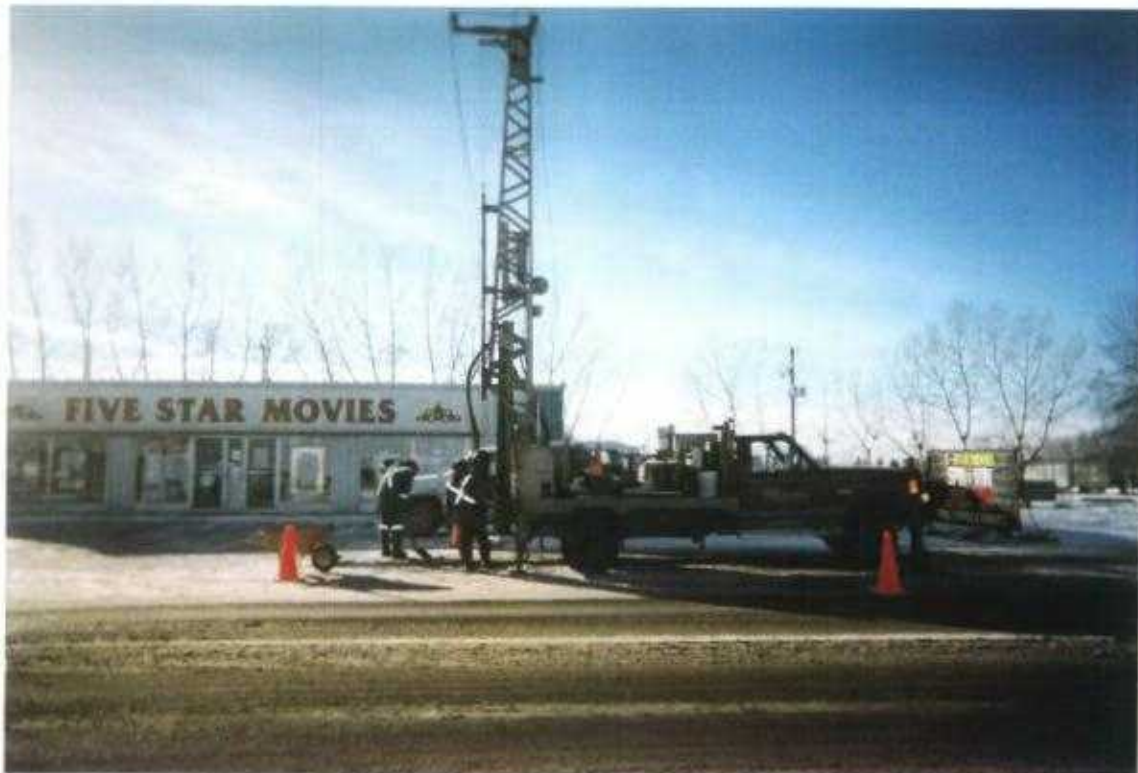
Photo No. 6 January 15 & 16, 2003; Phase III: Hydrocarbon ESA-Delineation Lots 5 & 6, Block 28, Plan 3845 CO; 419 - 10 Avenue, Carstairs, Alberta Looking West. Drilling Borehole #14.
