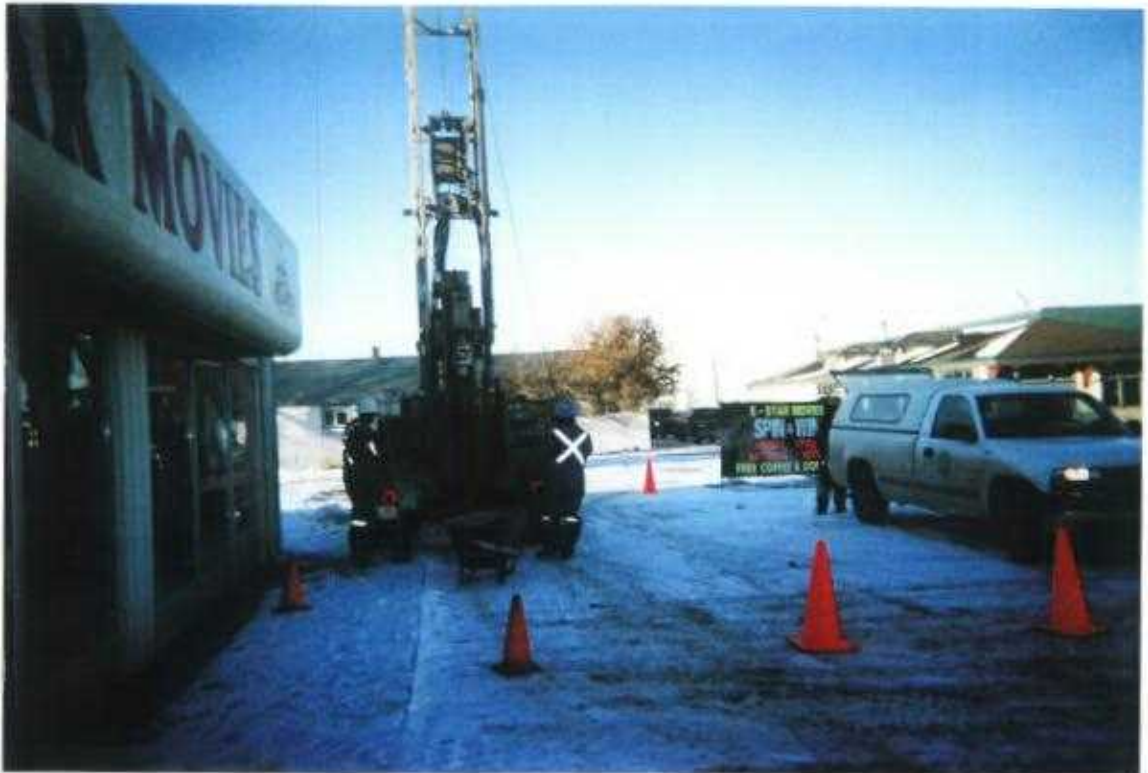
Photo No. 8 January 15 & 16, 2003; Phase III: Hydrocarbon ESA-Delineation Lots 5 &6, Block 28, Plan 3845 CO; 419 - 10 Avenue, Carstairs, Alberta Looking North. Drilling Borehole #16/Monitoring Well #5.
