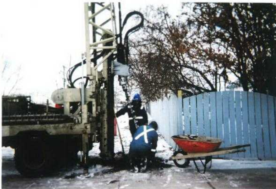
Photo No. 4 January 15 & 16, 2003; Phase III: Hydrocarbon ESA-Delineation Lots 5 & 6, Block 28, Plan 3845 CO; 419 - 10 Avenue, Carstairs, Alberta Looking West. Drilling Borehole #12/Monitoring Well #4.
