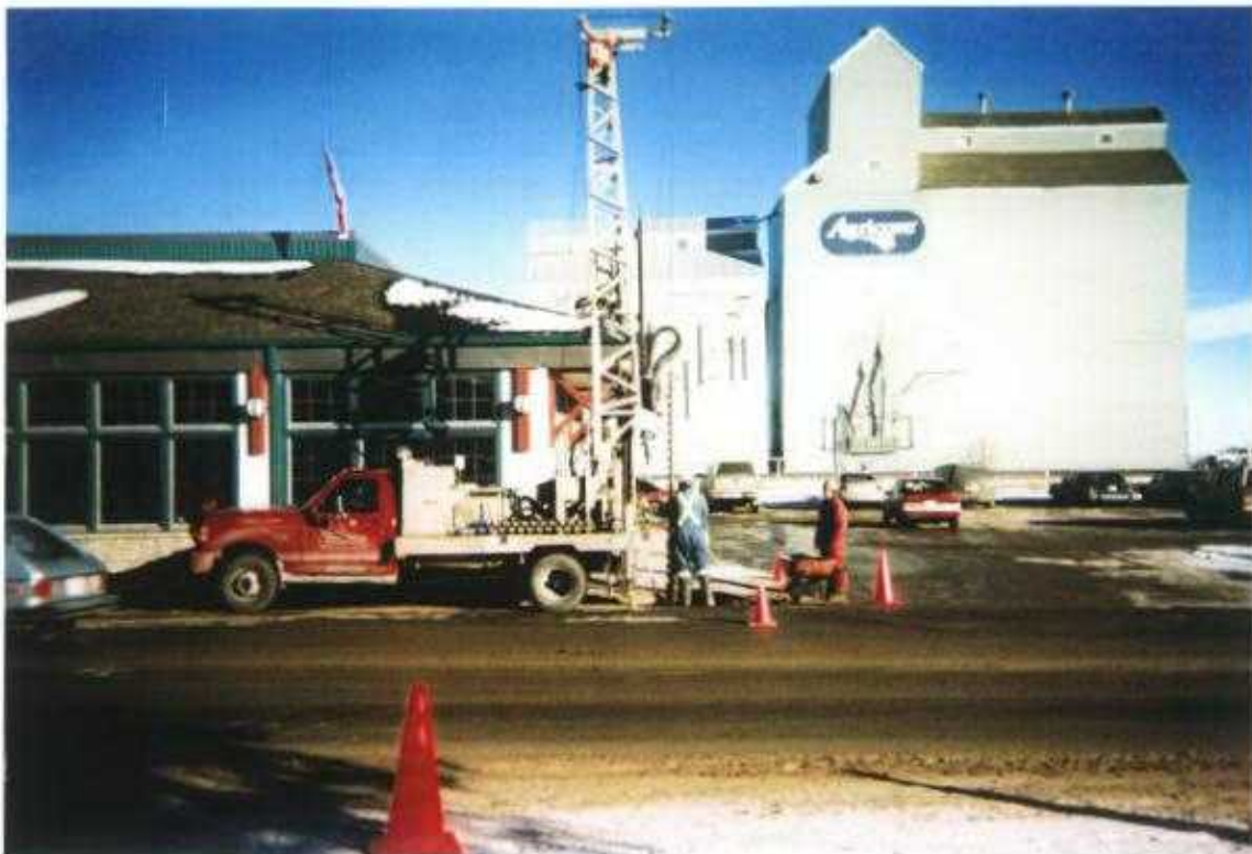
Photo No. 13 January 15 & 16, 2003; Phase III: Hydrocarbon ESA-Delineation Lots 5 & 6, Block 28, Plan 3845 CO; 419 - 10 Avenue, Carstairs, Alberta Looking East. Drilling Borehole #23/Monitoring Well #6.
