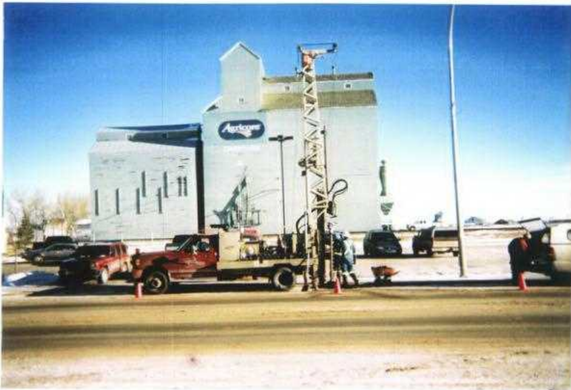
Photo No. 12 January 15 & 16, 2003; Phase III: Hydrocarbon ESA-Delineation Lots 5 & 6, Block 28, Plan 3845 CO; 419 - 10 Avenue, Carstairs, Alberta Looking East. Drilling Borehole #22.
