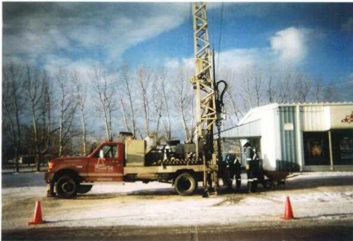
Photo No. 10 January 15 & 16, 2003; Phase III: Hydrocarbon ESA-Delineation Lots 5 & 6, Block 28, Plan 3845 CO; 419 - 10 Avenue, Carstairs, Alberta Looking West. Drilling Borehole #18.
