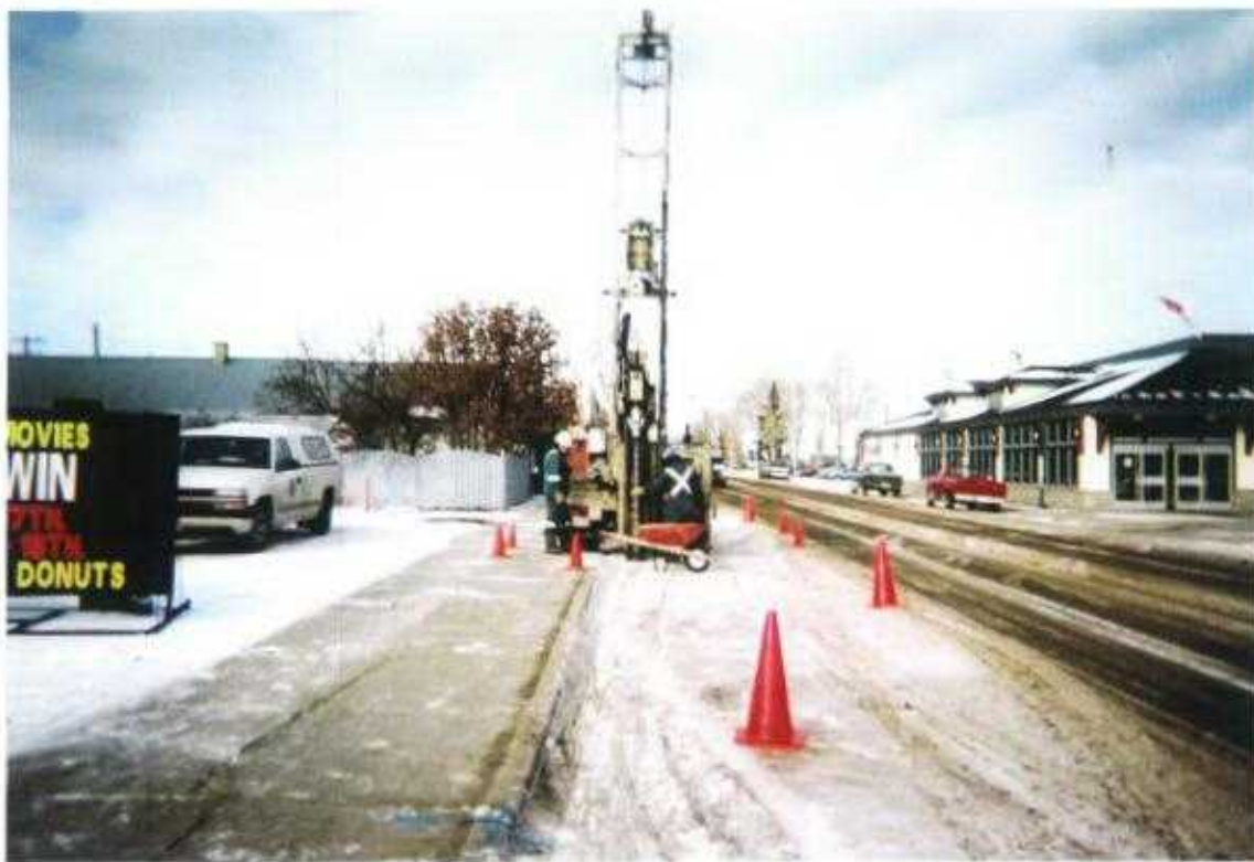
Photo No. 5 January 15 & 16, 2003; Phase III: Hydrocarbon ESA-Delineation Lots 5 & 6, Block 28, Plan 3845 CO; 419 - 10 Avenue, Carstairs, Alberta Looking North. Drilling Borehole #13.
