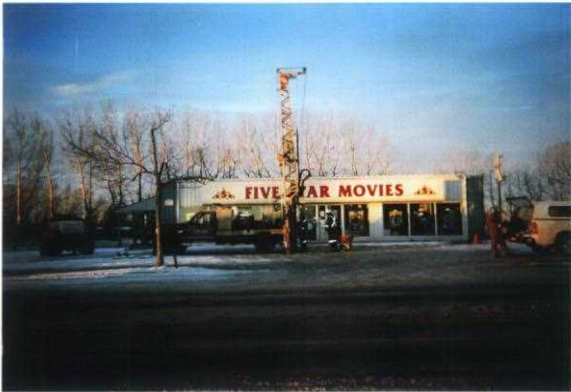
Photo No. 9 January 15 & 16, 2003; Phase III: Hydrocarbon ESA-Delineation Lots 5 & 6, Block 28, Plan 3845 CO; 419 - 10 Avenue, Carstairs, Alberta Looking West. Drilling Borehole #17.
