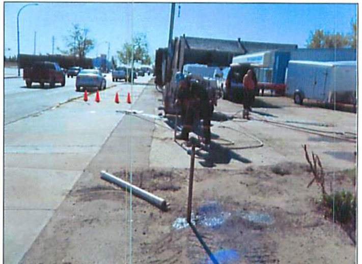
PHOTO 3 View of rig and nutrient injection points facing south.
